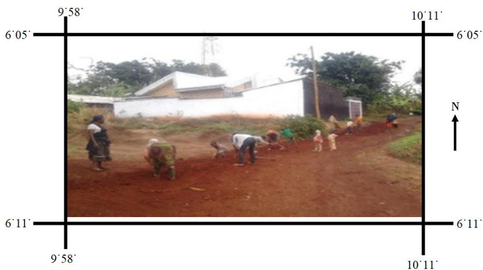
Plate 1. CBO led community labour in the laying of water pipeline in Manka'a, Bafut municipality in 2012
