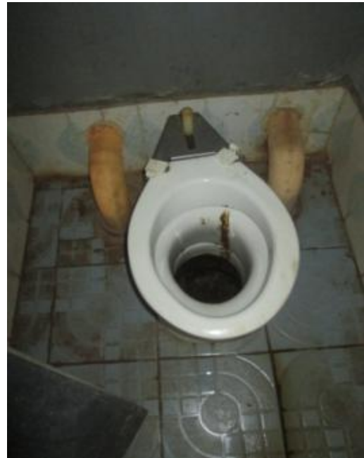
Fig. 5. Littered floor of the toilet
