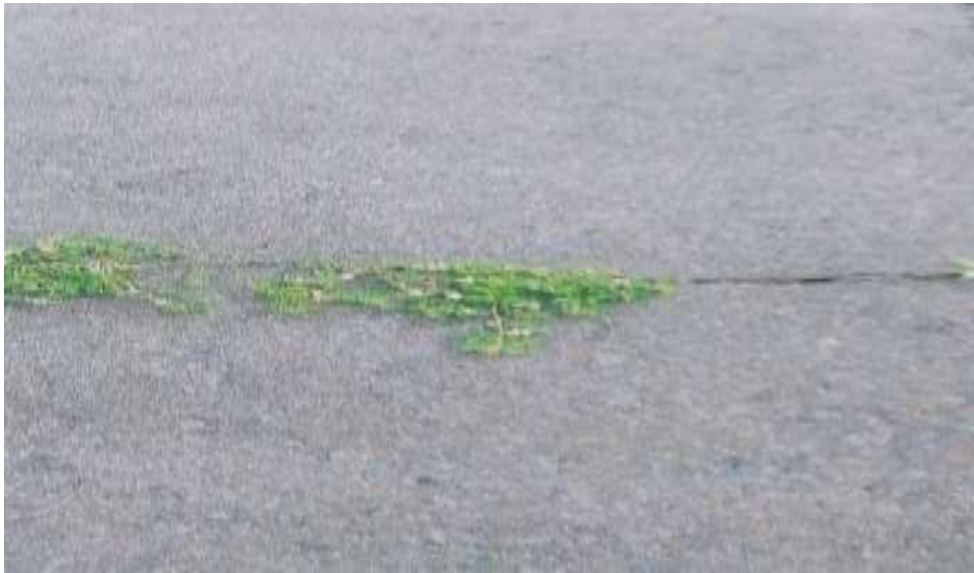
Fig. 7. Vegetation and grass growth in the cracks of in situ concrete
