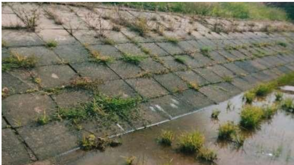
Fig. 6. Vegetation and grass growth on the joints of precast concrete
