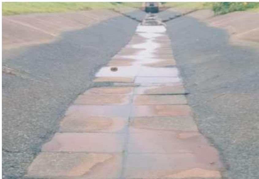
Fig. 4. Differential movements on the precast concrete
