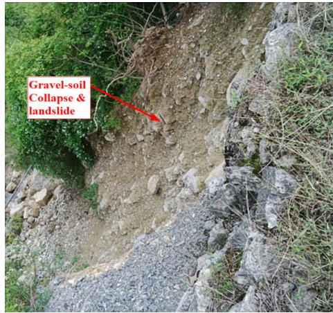
(b) Collapse and landslide of the gully bank in the circulation area
