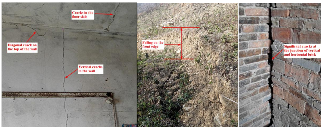
Fig. 9. Photo of house wall cracking and falling front edge within the range of Lijiadagou 1# landslide
