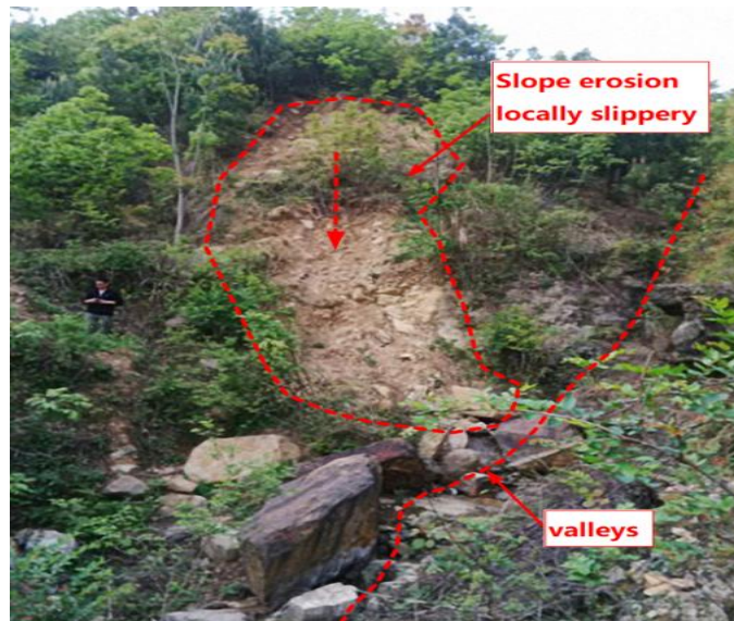
Fig. 6. Slope erosion and local slippery
