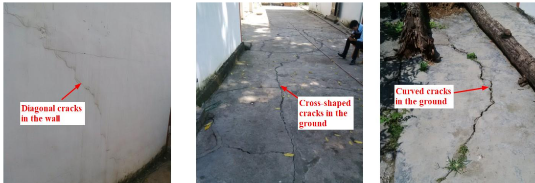
Fig. 11. Deformation of houses and roads within the range of Linjiawan landslide
